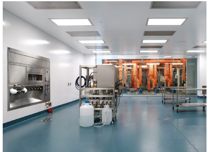
Utility access is via the stainless panel within the purification suite; heating hot water pipes color-coded orange appear across the viewing corridor in the mechanical area.
