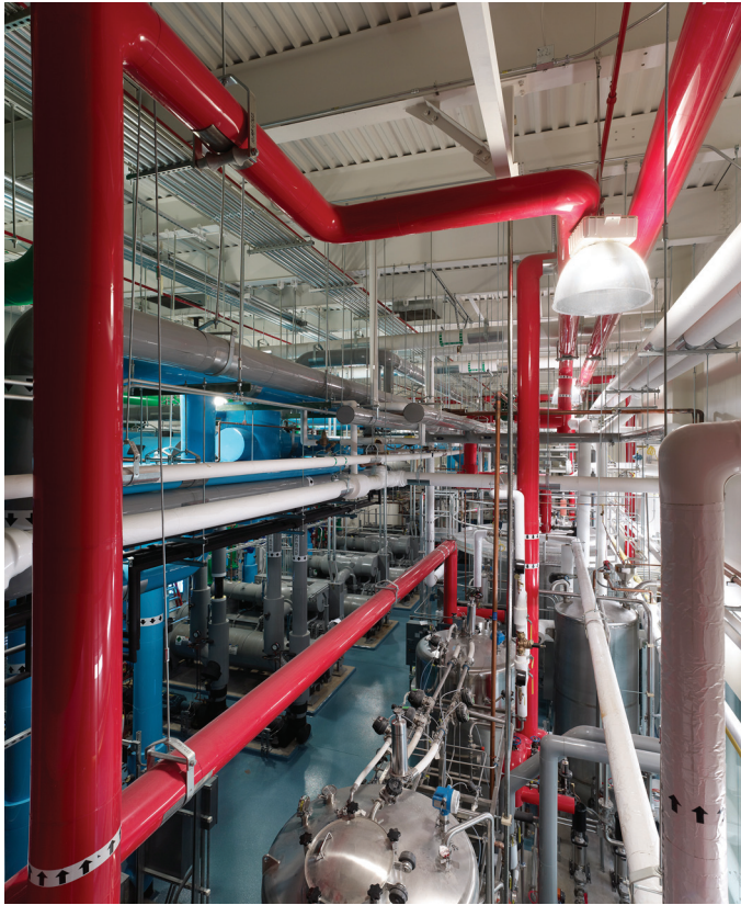
Completed mechanical room.
