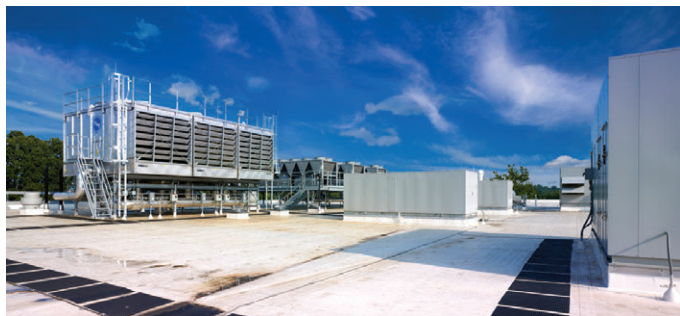
Pilot plant's rooftop includes air-handling units for each production suite; white roofing helps reduce the heat island effect.
