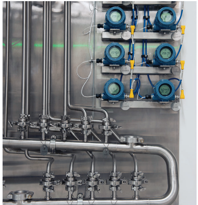
Bioreactor SIP piping.
