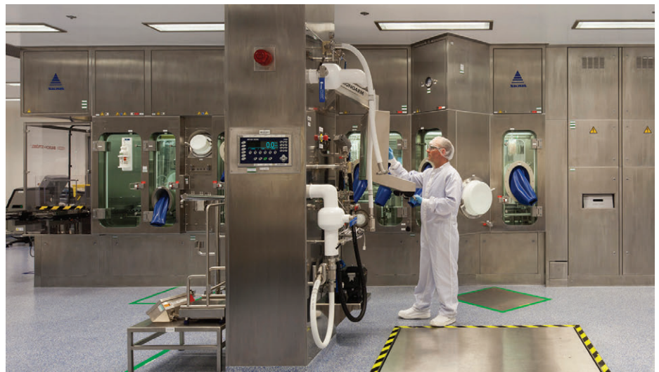
Operating interface for filling line.
