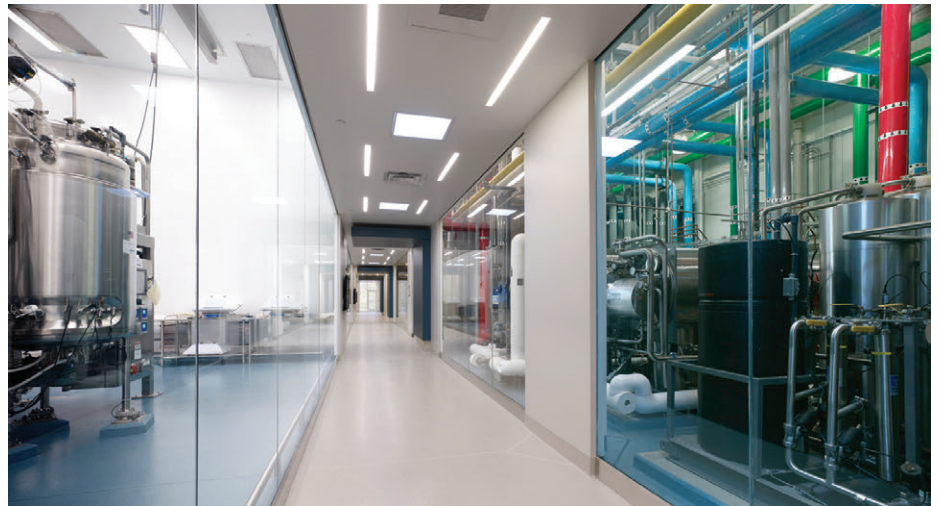
Glass-walled viewing corridor exposes production suites (left) and mechanical spaces (right); light tubes bring natural daylight into the corridor from above.
